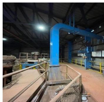
Fumes Absorber in Chemical Tank
